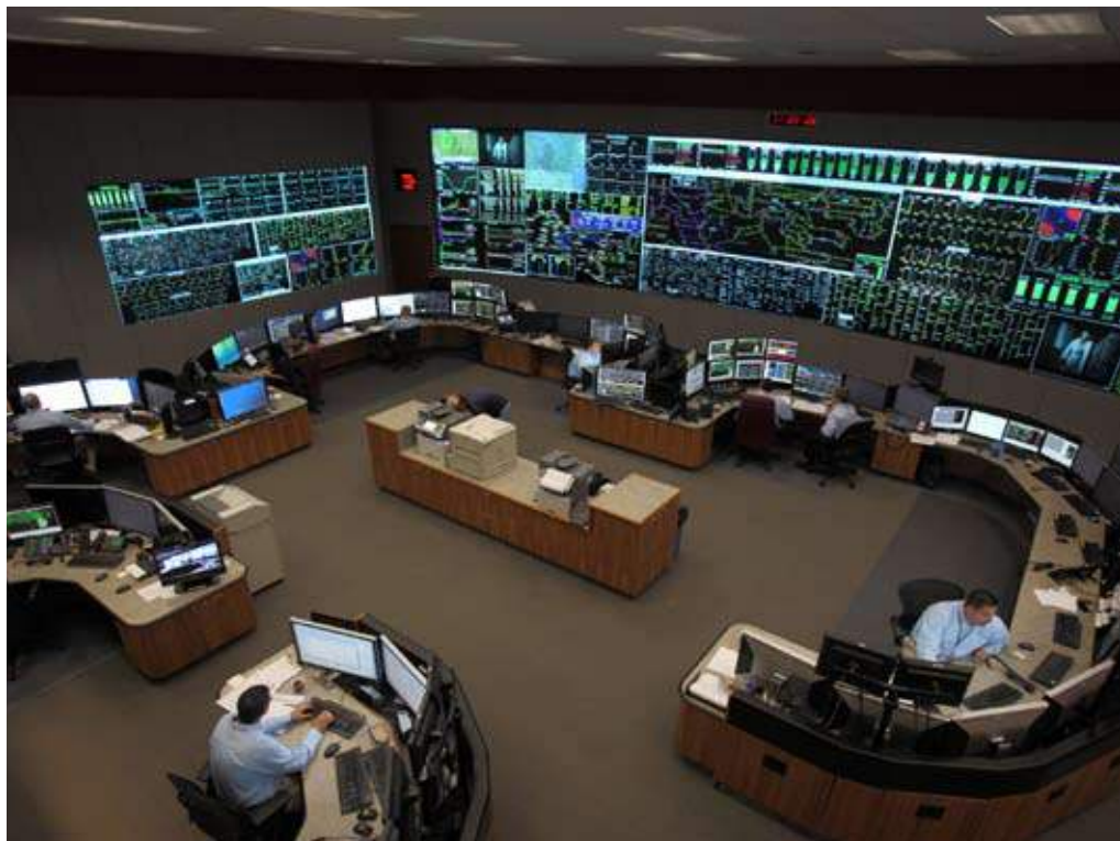
PJM Control Room - PJM © 2012. All rights reserved.
