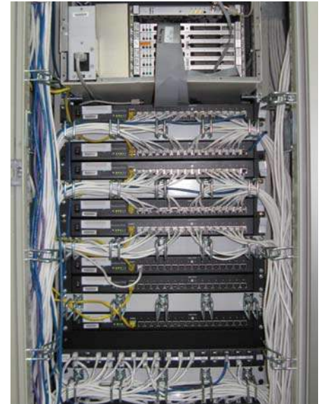
Front End Communication Devices and Cabling – TS16s and VME Chassis
