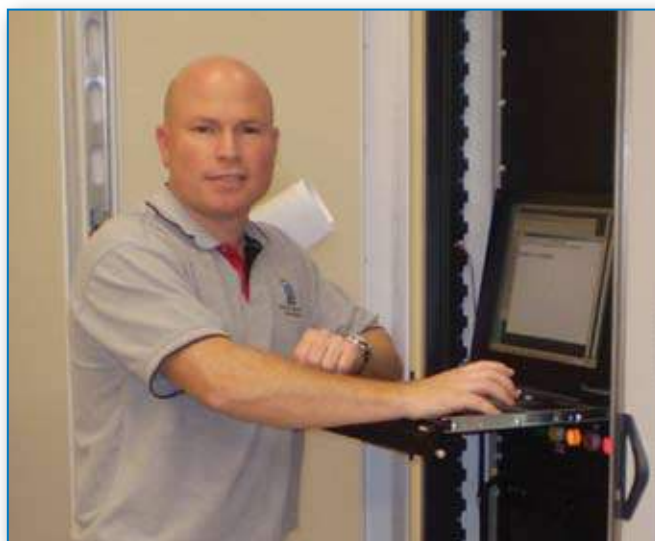
Kent Horan carries out testing on a control cubicle for the Apollo HVDC project
