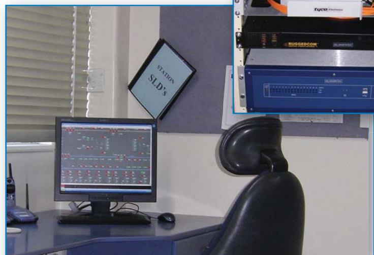
Islington Substation control desk and HMI equipment cabinet
