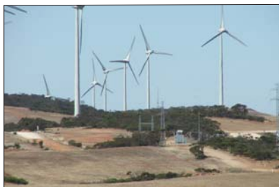
Mt Millar substation on the Eyre Peninsula in South Australia, surrounded by the Mt Millar Wind Farm
