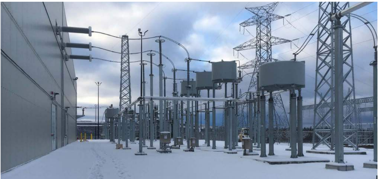
Maritime Link switchyard equipment at Bottom Brook substation
