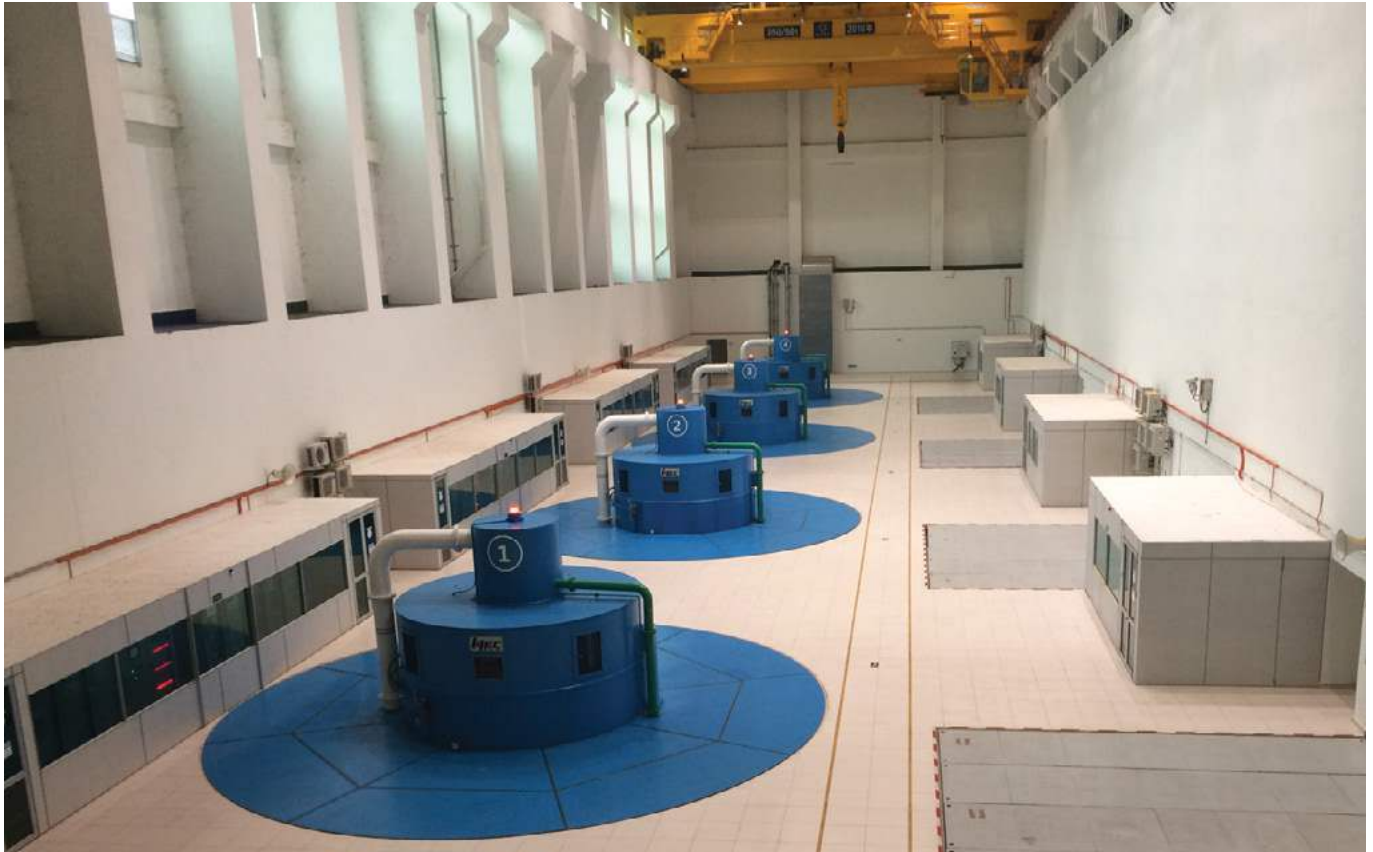
Murum HEP generator floor
