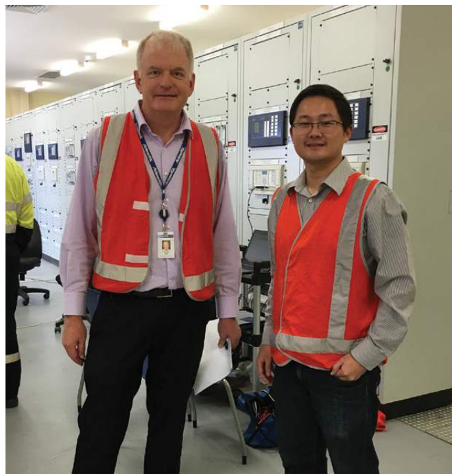
Testing being undertaken at an ActewAGL substation in Canberra. James Cole (L) – ActewAGL Secondary Systems Manager; Victor Tan (R) – PSC Principal Network and Security Consultant
