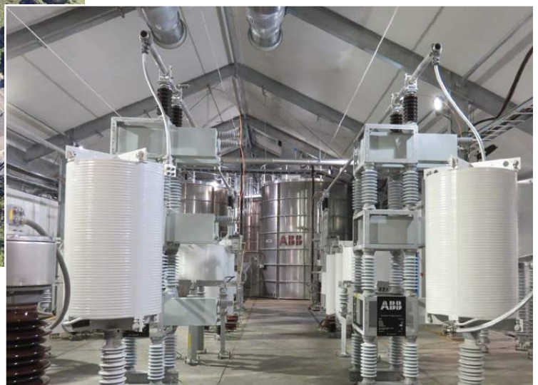
A view inside the new system 1 converter building
